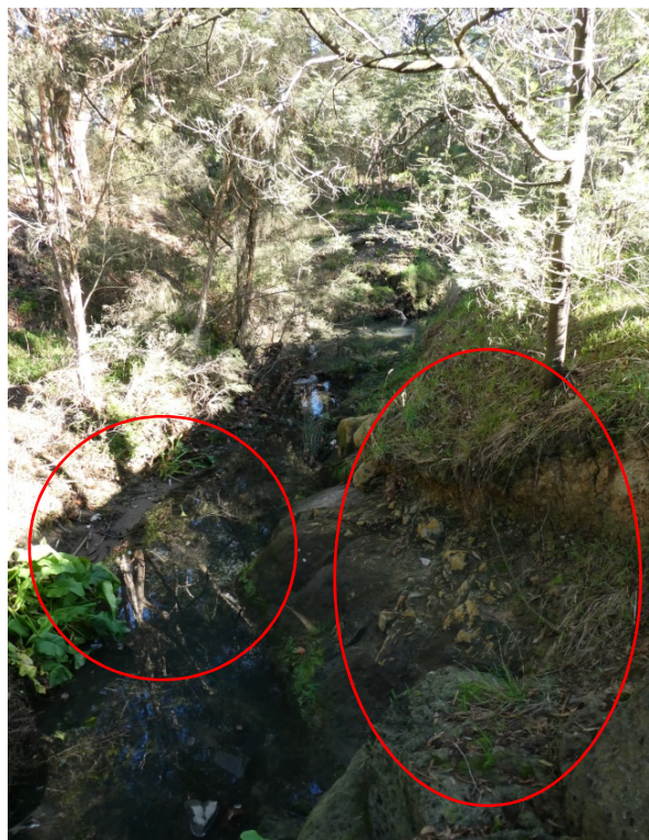
Erosion in the Glen Waverley Drain
