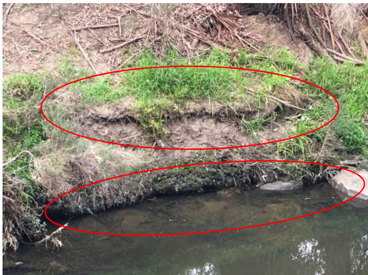
Slumping and undercutting at Regent Street
